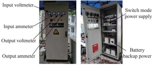
Figure 5 Actual power supply unit
