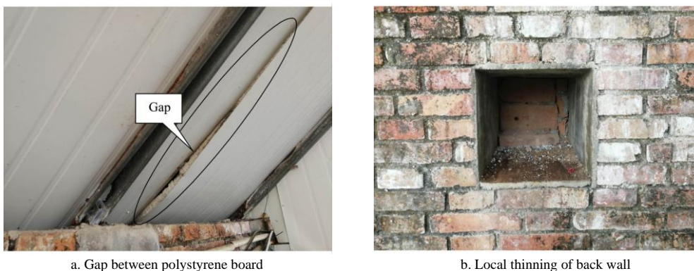
Figure 2 Photos of the prefabricated thermodynamic disfigurement (a) Gap between polystyrene board; (b) Local thinning of back wall
