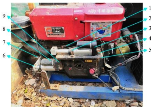
Figure 9 Actuator of diesel engine throttle and pressure reduction valve
