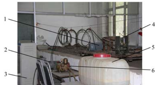
1. Motor 1 2. Motor 2 3. Frequency conversion cabinet 4. Intermittent type distributor 5. Liquid tank 6. Hydraulic pump
