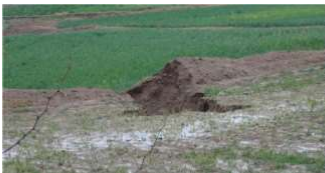
Figure A2 Breached terrace bund/embankment
