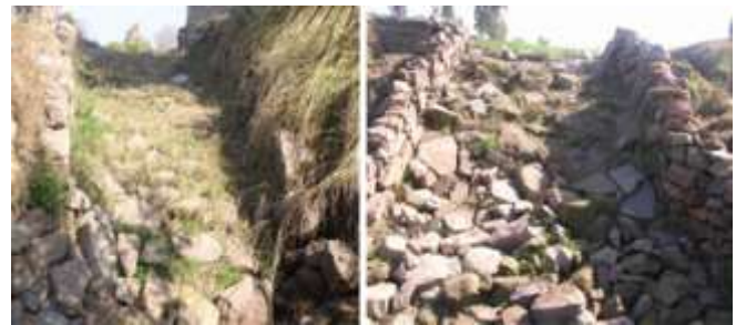
Figure A5 Front view of conservation structure built using local available stones
